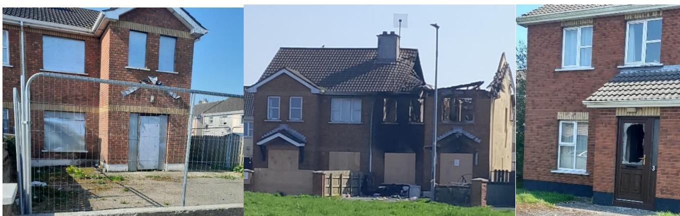
3: Photographs of boarded, derelict and damaged properties 12 April 2025
