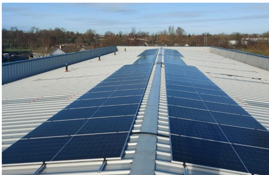
Photo 2 Solar PV on the roof of Longford Athletics Club.
