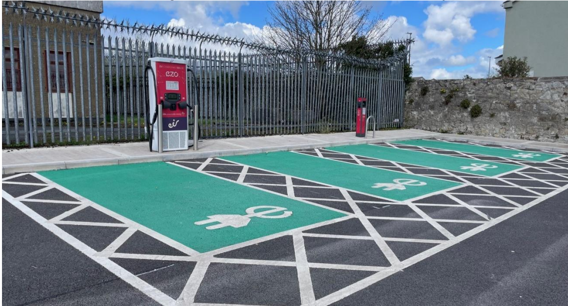
Photo 15 EV charging points in Granard
