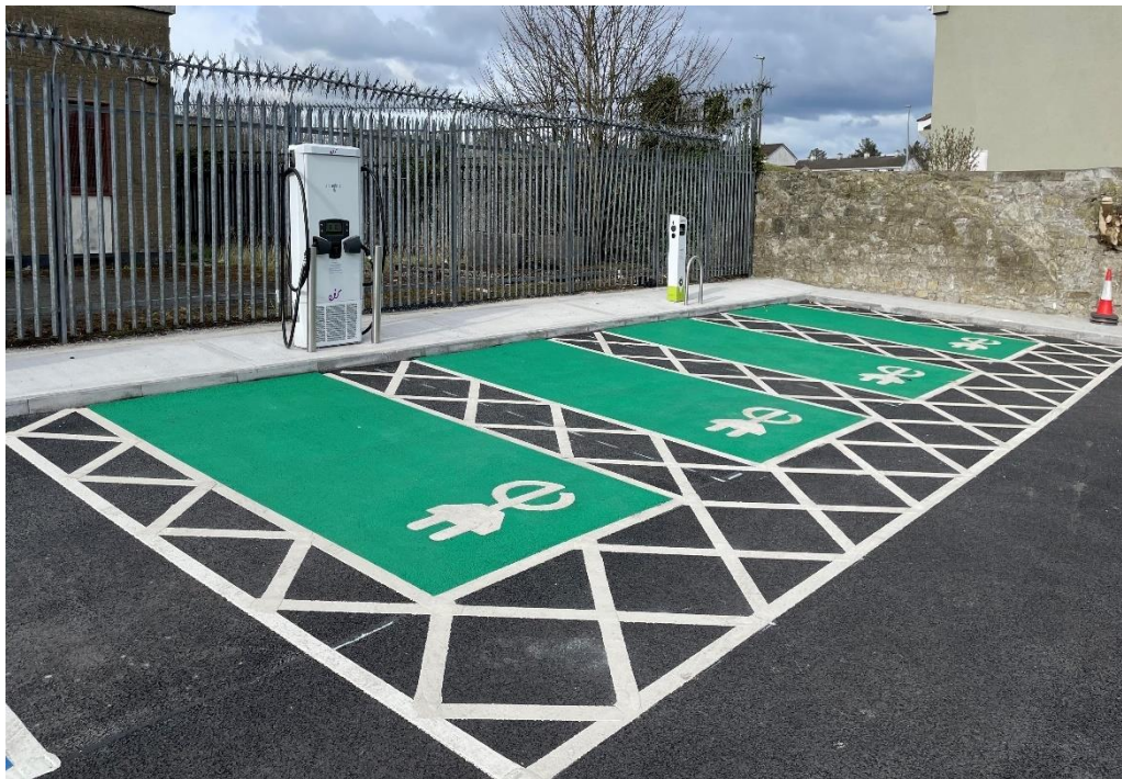
Photo – New EV charging station in Barrack Lane carpark, Granard.
