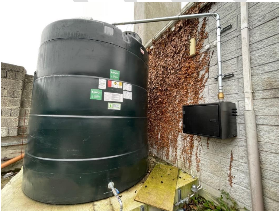
Photo 25 - New HVO tank as Aras an Chontae
