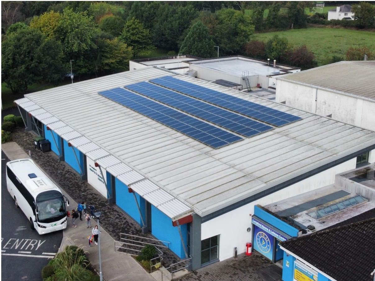
Photo 16 Solar PV panels at LONGFORD SPORT & Leisure Centre
