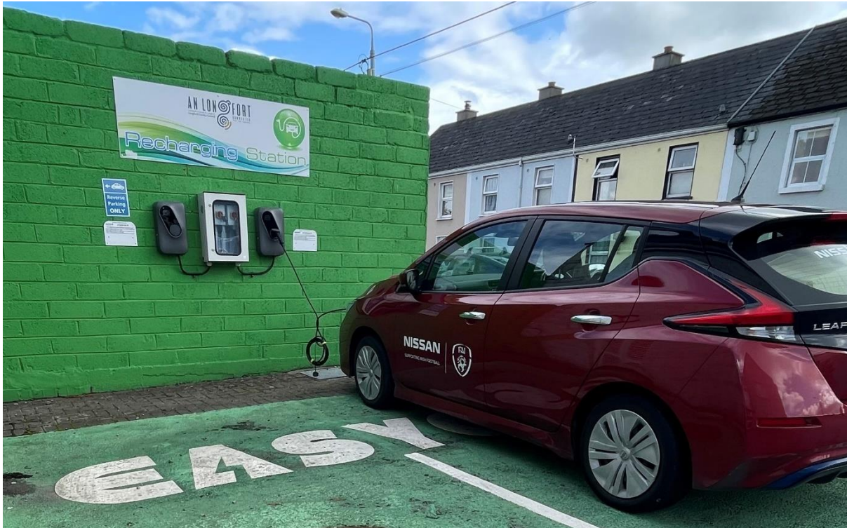
Photo 17 EV Charging Station at Arás an Chontae, Great Water Street, Longford
