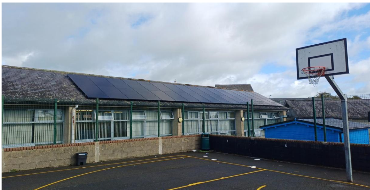
34 Solar Panels installed at St Josephs N.S. Longford.
