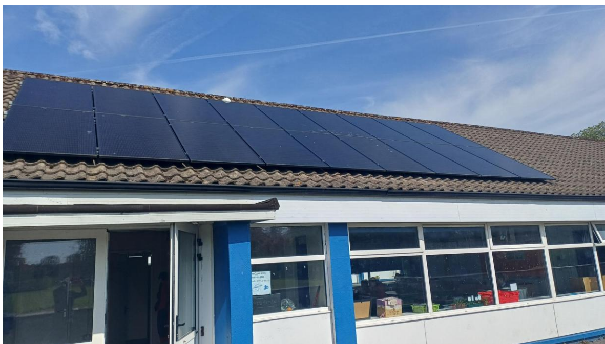
18 Solar Panels installed at St Michaels Boys N.S. Longford.
