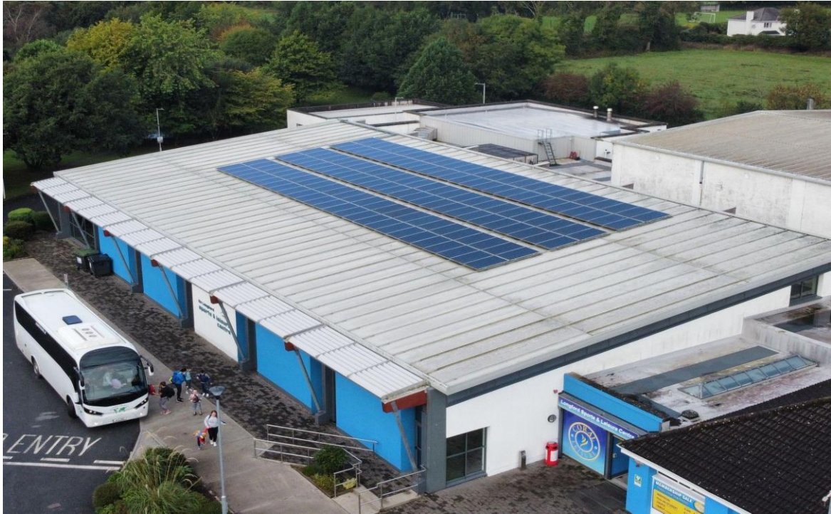
Solar Panels on Longford Leisure Centre.
