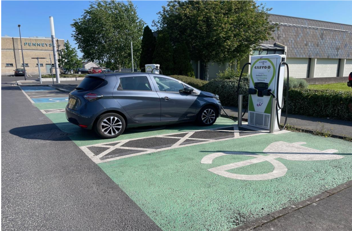
New 75KW Electric Vehicle Charging Points installed at the Public Library in Longford Town.
