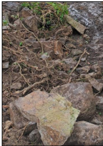
Plate 6: Stone from break in the wall
