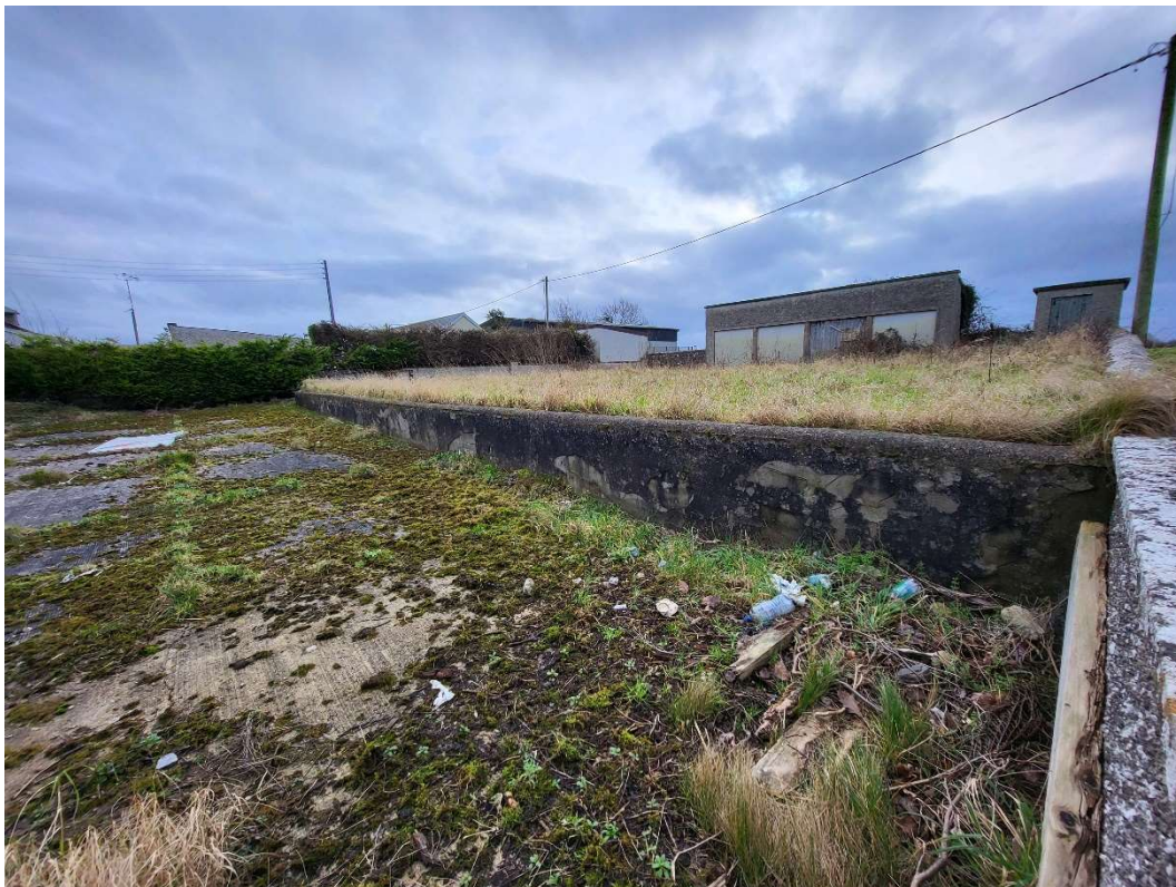
KLA – Image of playground shelter and outbuilding to rear of Scoil Náisiúnta Naomh Colmcille
