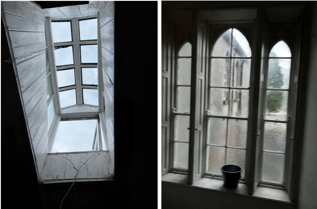
KLA – Image of original timber rooflights which are in severe disrepair & first floor feature window in the Convent of Mercy
