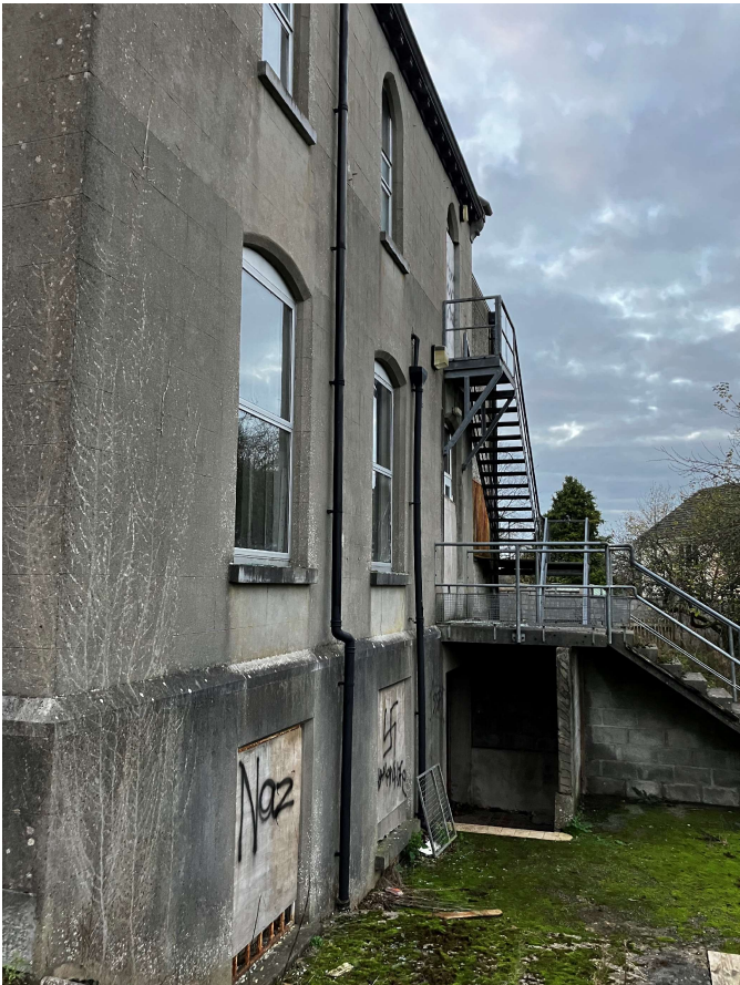
KLA – Image of external stairs to be demolished on east side of building
