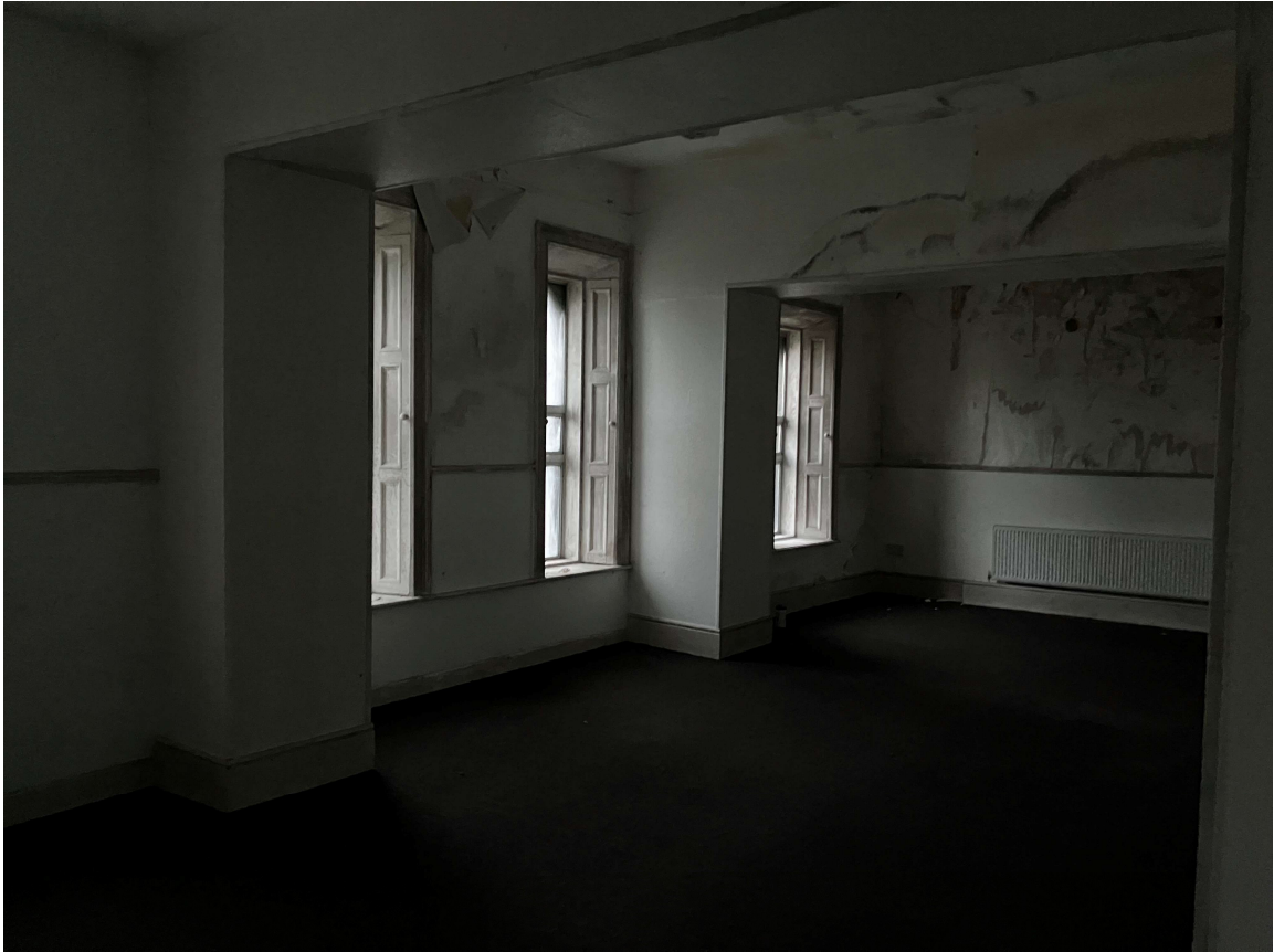
KLA– Image of the extensive water damage and damp on the upper floors
