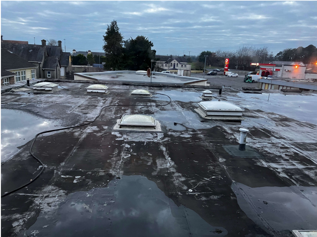
KLA – Image of flat roof extension to southwest of Convent, with hexagonal extension in background
