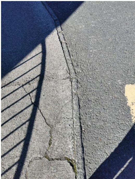
Lack of tactile paving at crossing
