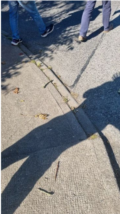
Lack of tactile paving at road crossing
