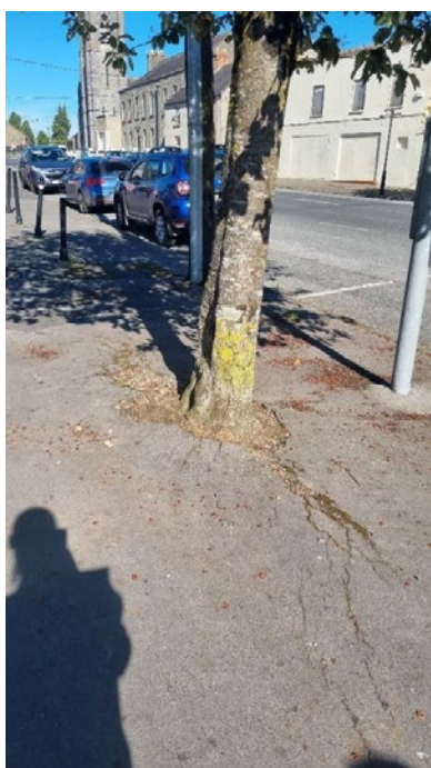
Tree uprooting pavement
