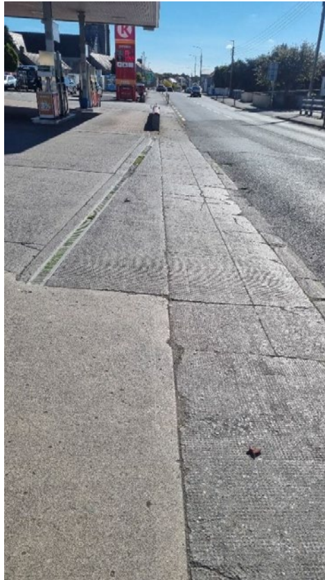
Lack of priority for pedestrians and conflict at entrance
