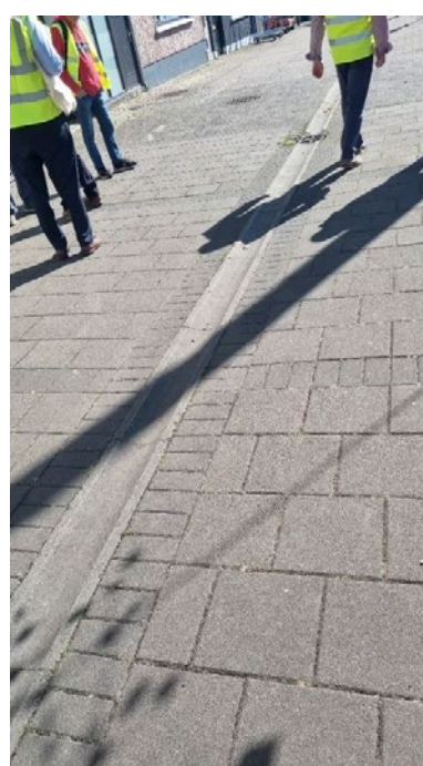
Channel drain within footpath
