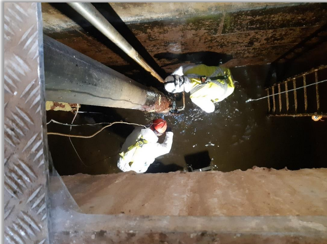
Longford County Council Water Services staff at work in a designed confined space with rescue equipment in place.
